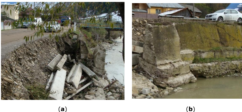
Figure 4. Details regarding the mode of degradation of the bank defence at research point P1: (a) – total destruction of the retaining wall and the advance of the riverbed into the road structure; (b) – stages of degradation of the retaining wall, with its displacement from the site (Luca, 2016).
