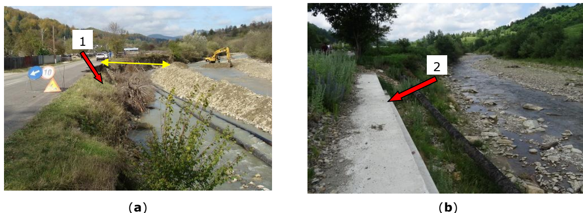
Figure 11. General view of the erosion of the right bank of the Tazlau Sarat River, research area P3: a – upstream view highlighting the erosion of the bank and the DC 180A road in 2016 (1 – remainder of the retaining wall); b – downstream view in 2019 of the riverbank defence rehabilitation work (2 – gabion wall located at the edge of the road) (photo author, Oct. 2019).
