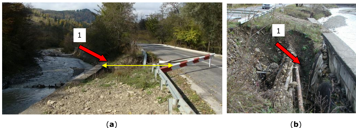
Figure 7. Details regarding the degradation of the bank defence at research point P4: (a) – erosion pit behind the retaining wall and the advance of the riverbed in the riparian area, 1 – erosion pit; (b) – hydraulic installations located in the river bank (Luca, 2016).
