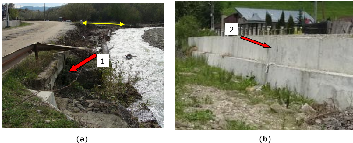
Figure 9. General view of the erosion of the left bank of the Tazlaul Sarat River, research area P2,: a – upstream view highlighting the destruction of the bank defence, year 2016 (1 - simple concrete retaining wall) and the degradation of the communal road DC 180A (Luca, 2016); b – downstream view of the new bank protection work (2 - gabion retaining wall) (Author's photo, 2019).
