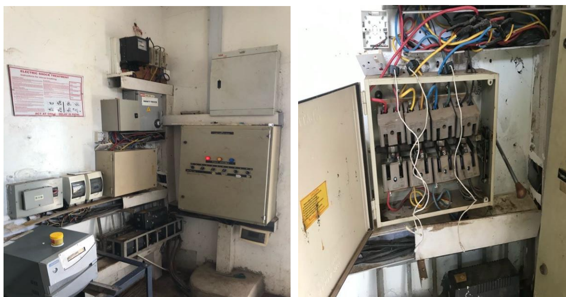
Figure 1. Pictorial view of the efergy with three Magnetic probes connected to the central load lines of the transfer switch in the admin block
